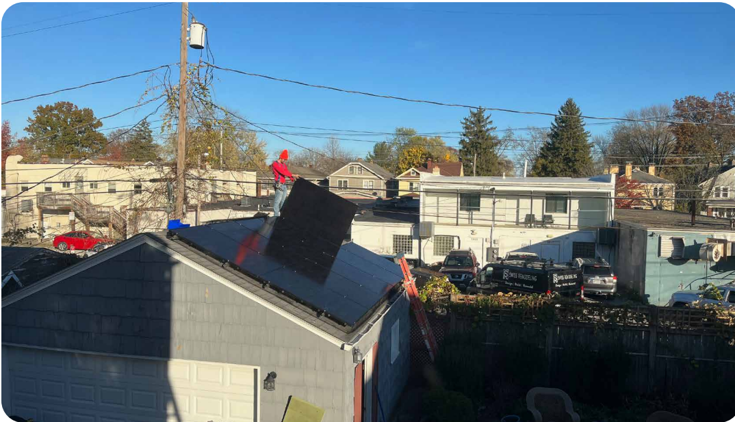
Solar energy system is installed on the roof of one of the households benefiting from the Low to Moderate Income Solar Co-op Pilot Program
