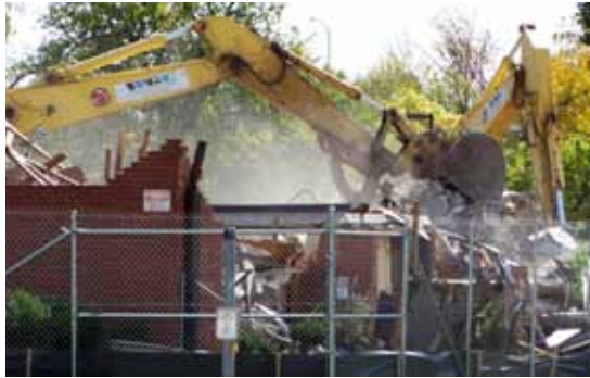
Demolition of the Riverside Bradley development contributed to the decline in plan-area population.
