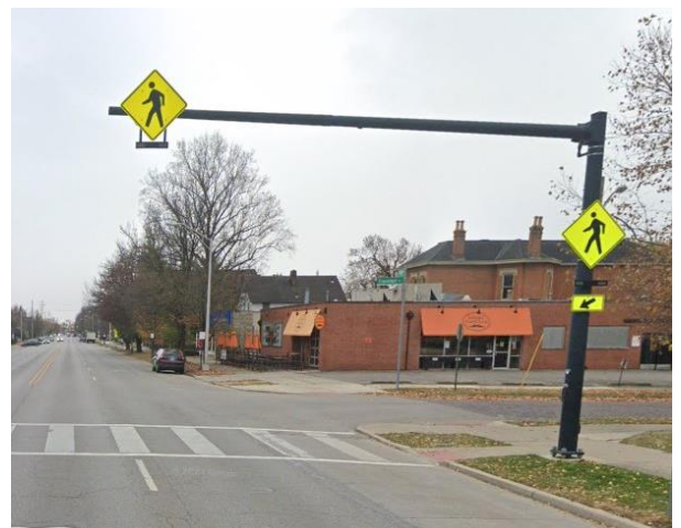
RRFB at High Street and Frankfort Street.
