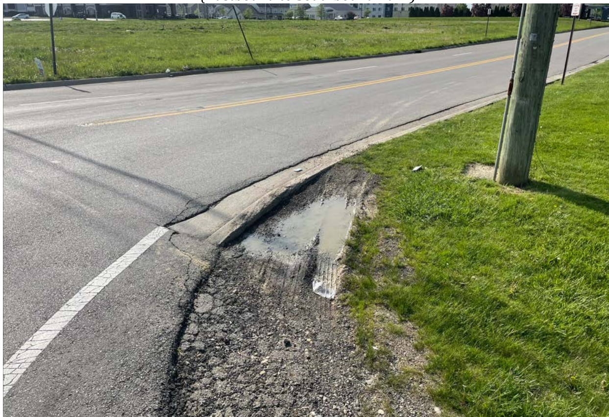
Figure 5 – Renner Road & W. St. James Lutheran Lane Southwest Corner (Eastbound to Southbound Turn)
