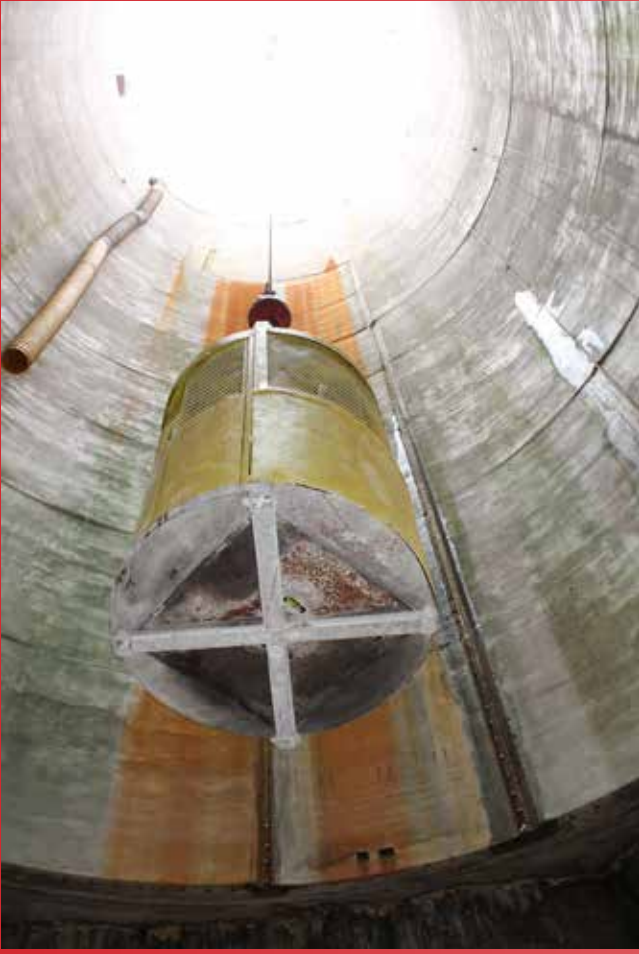
OARS tunnel shaft and transport cage
