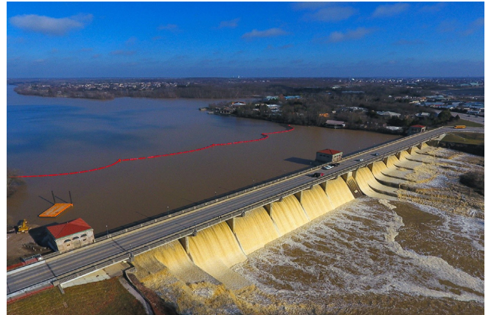
O'Shaughnessy Dam Spillway Improvements Project - Dam After Installation Of New Flashboards, Debris Boom, And Downstream Erosion Protection Repairs
