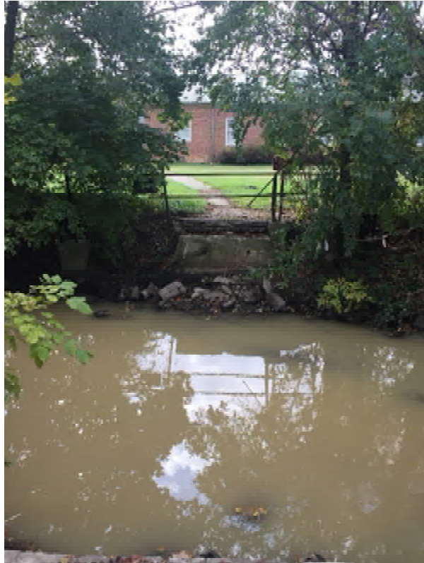
View of Collapsed Bridge Facing West
