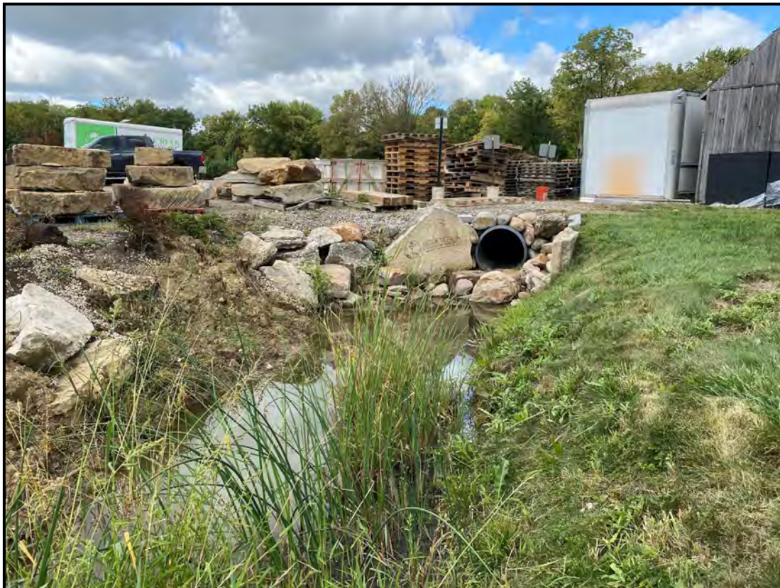
Photo 2 – Northwesterly (upstream) view towards the beginning of the assessed stream. The 200' evaluation area begins at the outfall of the culvert pipe shown near the center of the photo.
