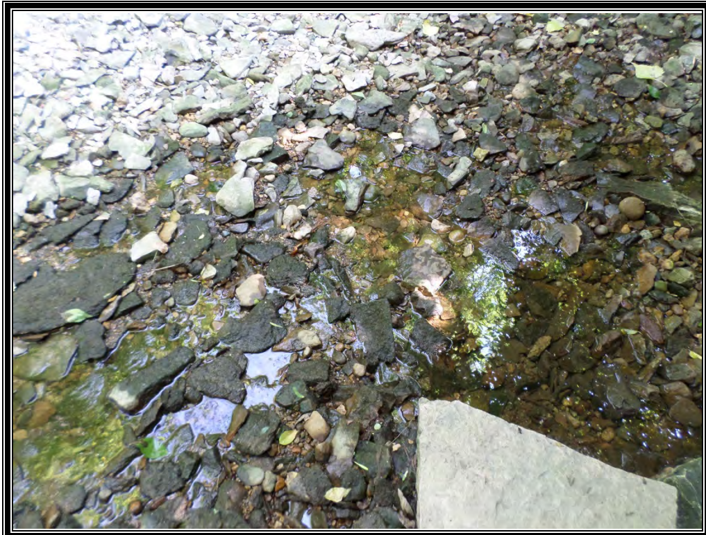
Photo 15 (6/14/16): Visible surface flow from the area seen in photo 14. Note the unconsolidated material comprising the bed of the man-made channel.
