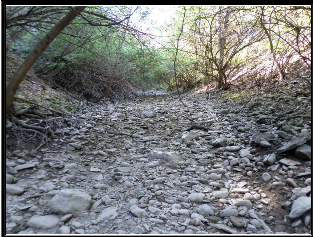
Photo 21 (4/20/16): View of the man-made channel on the west central portion of the property. This channel is located between a mine high wall and a steep berm.
