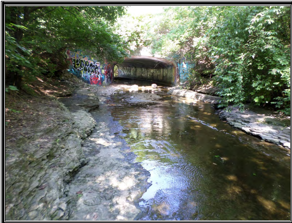
Photo 6 (6/14/16): Westerly (upstream) view of Roberts Millikin Ditch as it enters the site. Flow is over exposed limestone bedrock.
