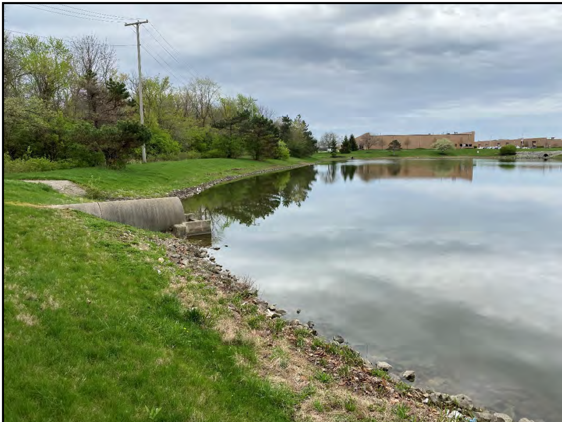
Photo 30 – Southwesterly view at the west adjoining storm water management pond directing surface water to Stream 9.
