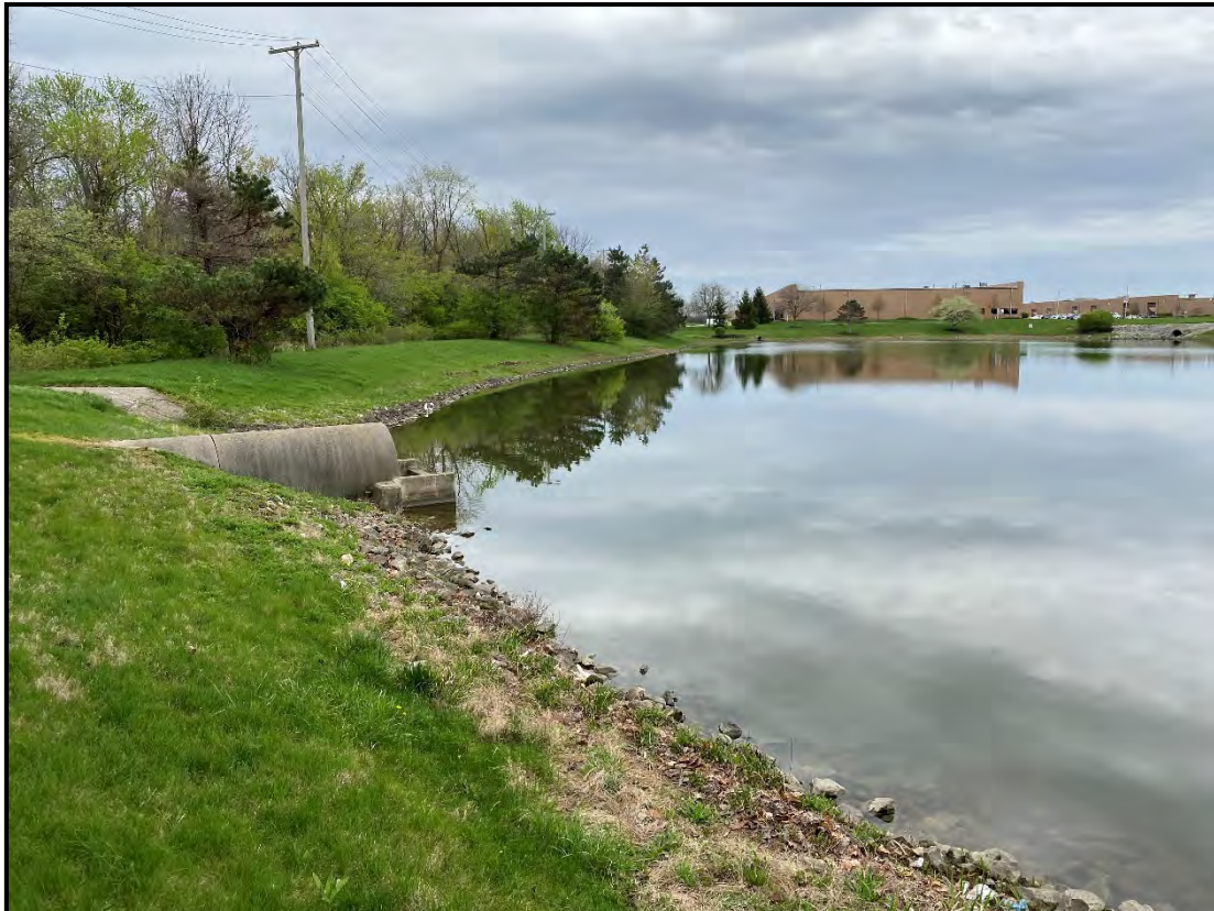
Photo 30 – Southwesterly view at the west adjoining storm water management pond directing surface water to Stream 9.
