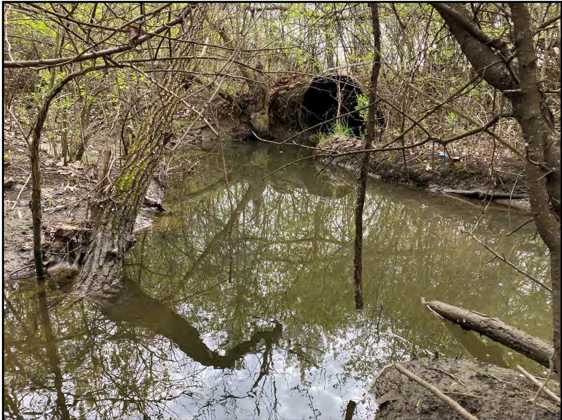
Photo 36 – Northeasterly view of the confluence of Stream 9 with Stream 10 on the northwest part of the Central Section of the evaluation area.
