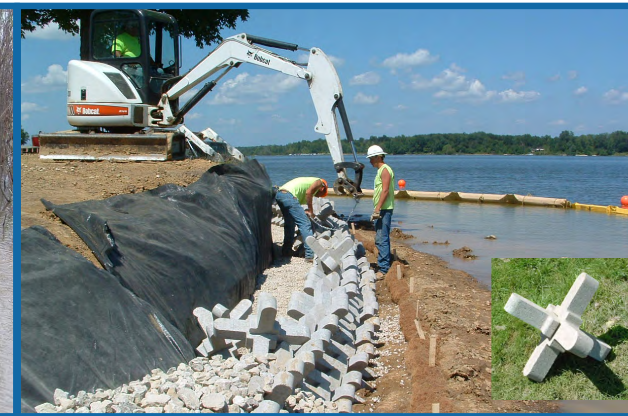
A-jacks® stabilizes severe bank erosion and allows interspersed plant growth for added protection.
