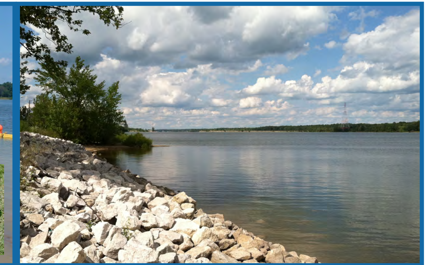
Rip-rap is a durable solution for protecting large areas of shoreline, preventing further erosion.
