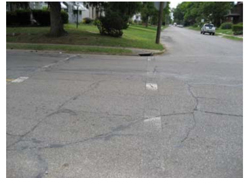
Faded crosswalks, children need to cross this intersection to get to school or the bus.
